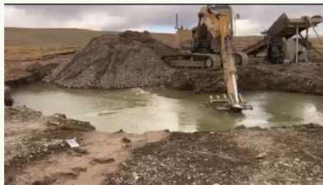
Mining excavator being used at the gold mining site in Kashi. Photo: Tibet.net
