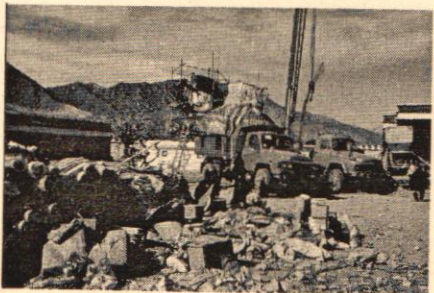
Under construction site of the Guru Padmasambhava statue at Samye Monastery before its demolition in May. The photo was taken in January by an unknown person. ©TCHRD
